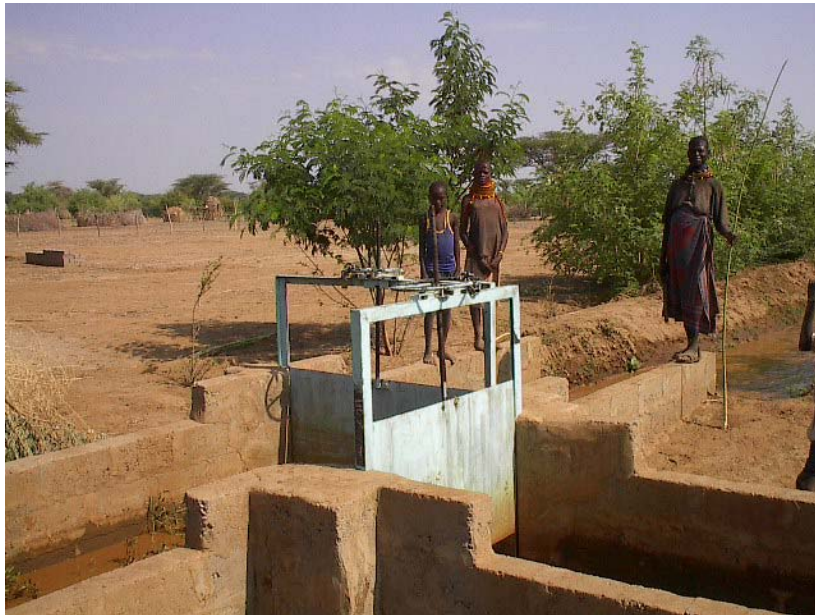
Picture 1: A division box in the Phase II part of the scheme. It clearly shows the lockable gates and cement re-enforcements to protect the canal banks.
