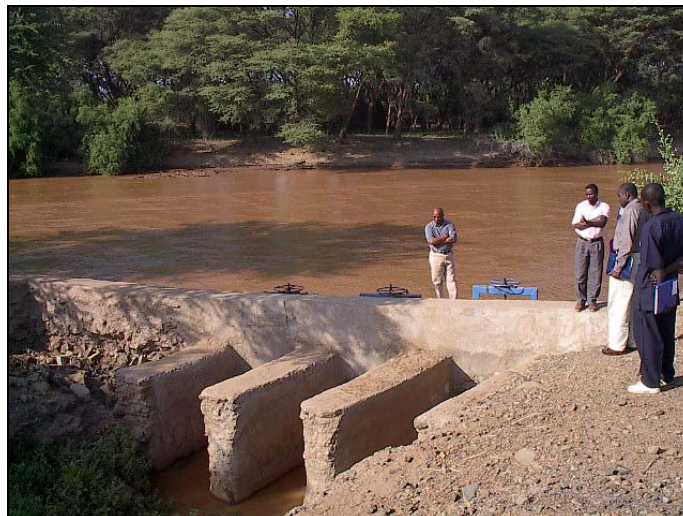
Picture 8: New intake constructed during Phase II (FY 1997-FY2001). Sustainability features include a settling-basin and back-flush mechanism to reduce siltation and maintenance work
